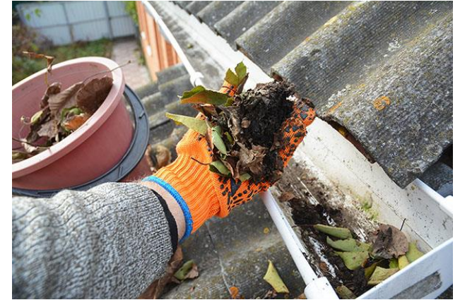
Regularly clean roofs and gutters!
